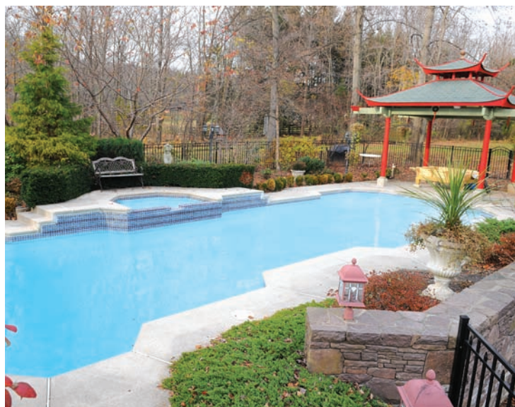
This pool's finish was starting to show its age. Carlton Pools applied AquaBright™ in Tahoe blue to give the water a beautiful Caribbean look.
